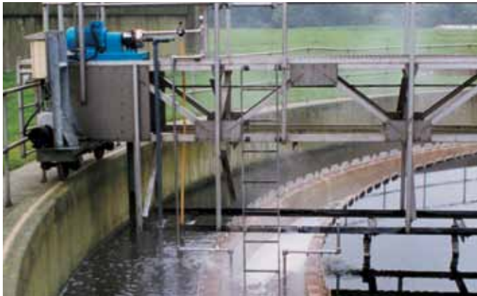
Wastewater treatment is a difficult pumping application that Hydra-Cell routinely handles.
