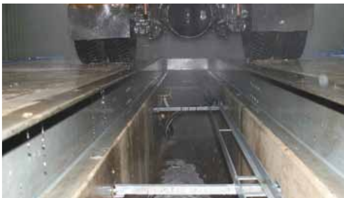
Pumping dirty and recycled water at a commercial car wash is an everyday function for Hydra-Cell pumps.
