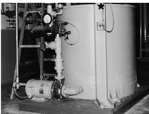
Reverse osmosis, Ósmosis invertida
